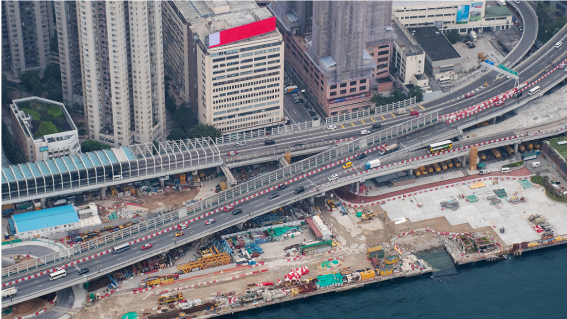
Figure 3 - Current condition of SNSE works between Piers 17 and 22 at IEC westbound bridge
