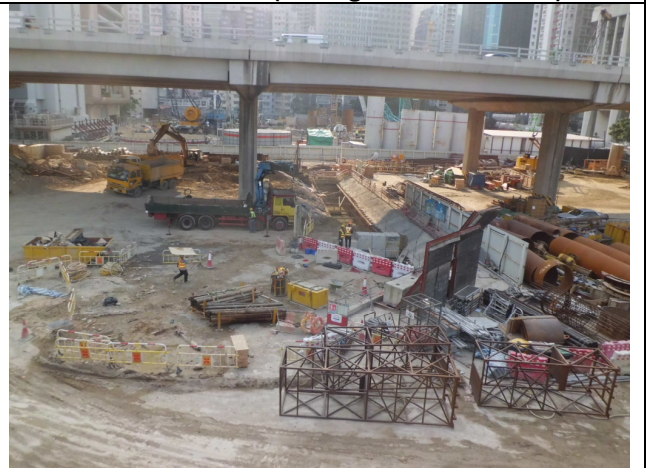
Photo 4 - Private Project Site to Harbour Grand HK Hotel (Wan Wah Mansion behind the Hotel)
